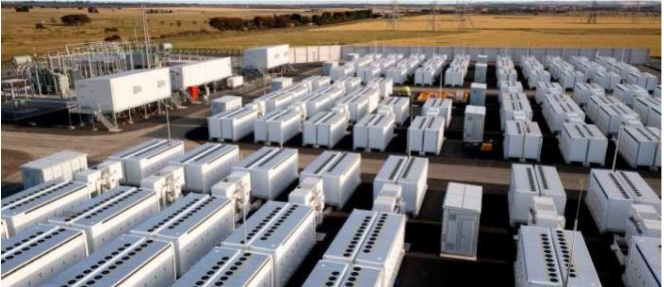
Photo 4.19 Example of a typical BESS (Wax Design, 2026; Victoria State Government, 2023)
