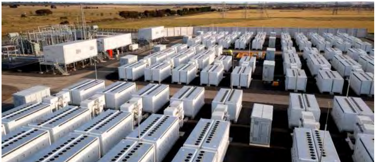
Figure 29: Image of typical layout of a BESS (Neoen-Tesla's Victorian Big Battery. Image: Victoria State government)
